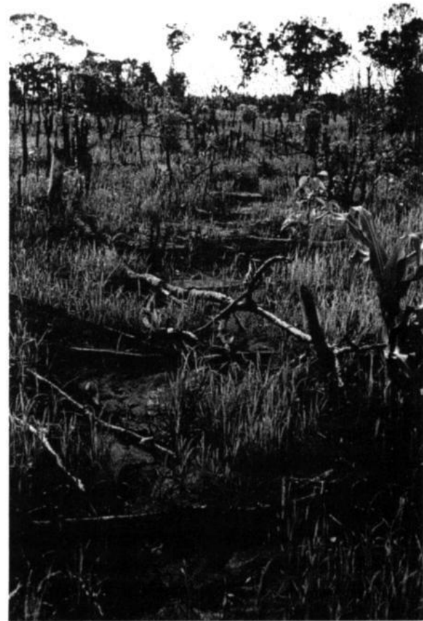
35. Construction of stick bunds across incipient gullies in a Sierra Leone rice field
