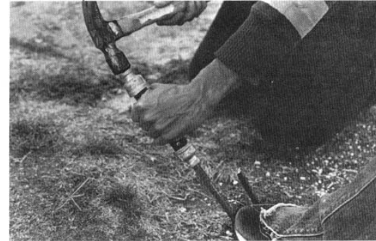
Place the driver over the sharpened end of the rebar stake and hammer it in.
